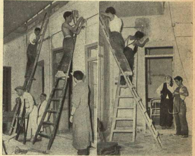
ORT Students installing Electricity in the Old Age Home at Ariana near Tunis
