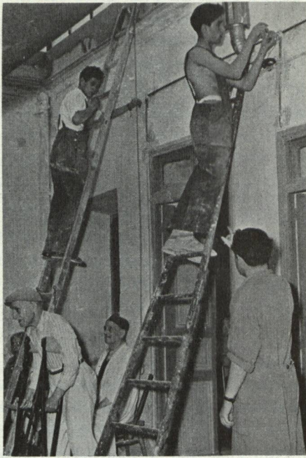
Upper class students at the Electrical School of the Tunis ORT Center install the first electrical facilities in the Tunis Home for the Jewish Aged.
